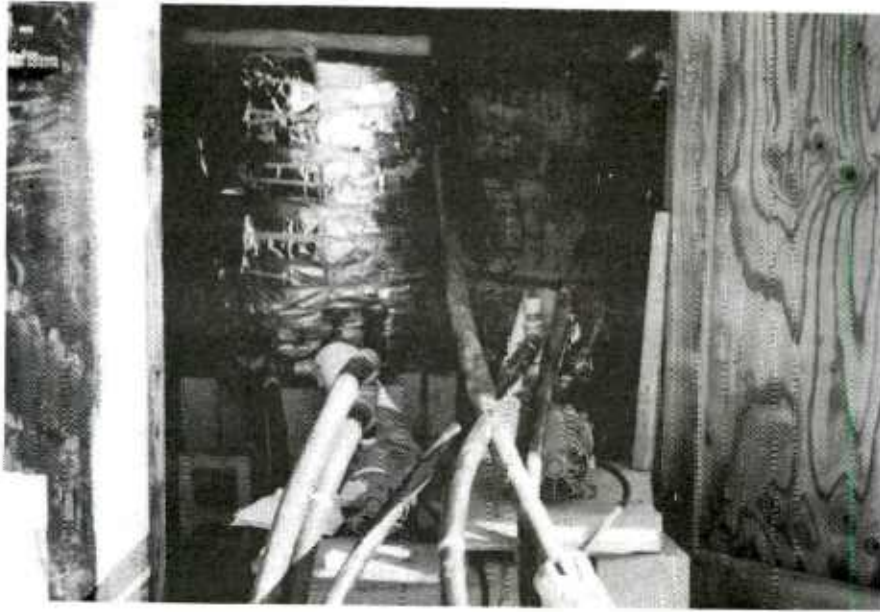
Fig 21 Hot and cold water reservoirs with corresponding hose and booster pumps
