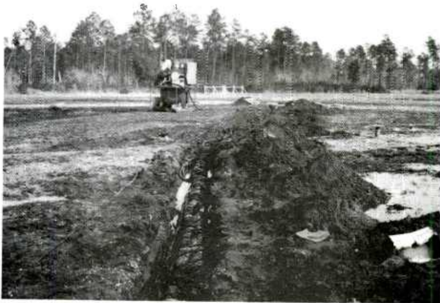
Fig 22 Insulated hose lines and electrical line layout
