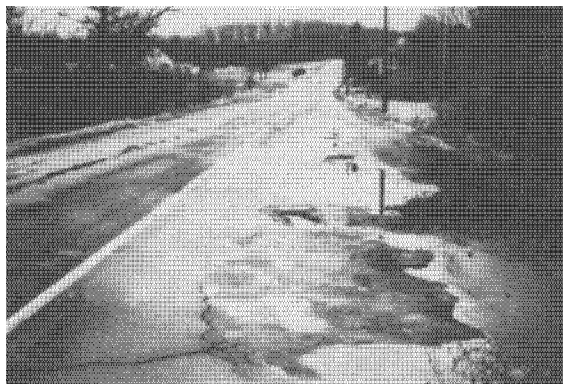
Poor shoulder maintenance traps water on road
