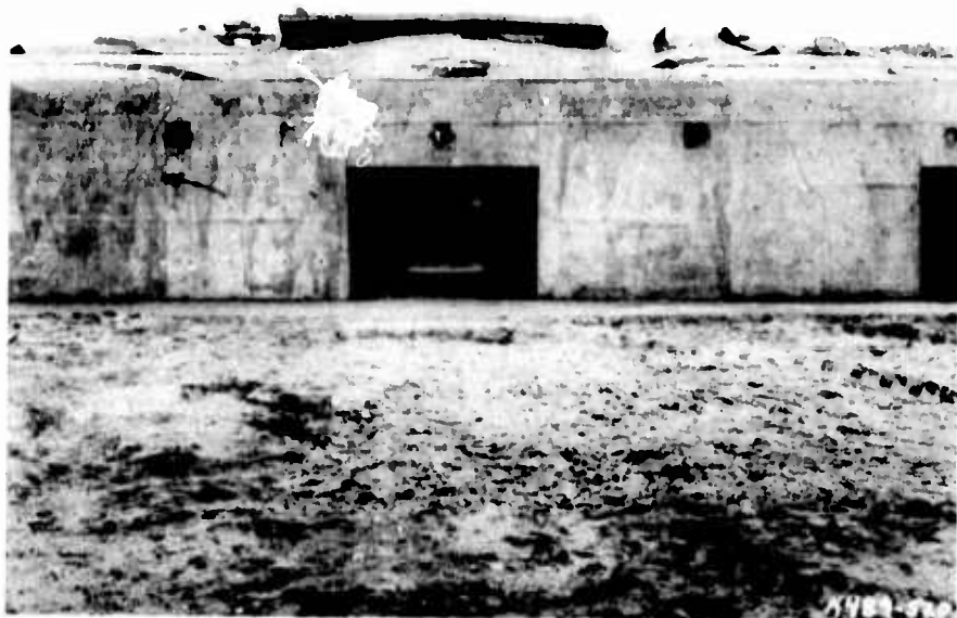
Figure 5.22. Posttest view of retaining wall after removal of ramp and debris.
