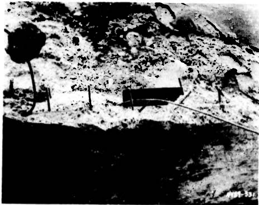
Figure 5.26. Damage to south part of donor bay air-lock blast door bulkhead.
