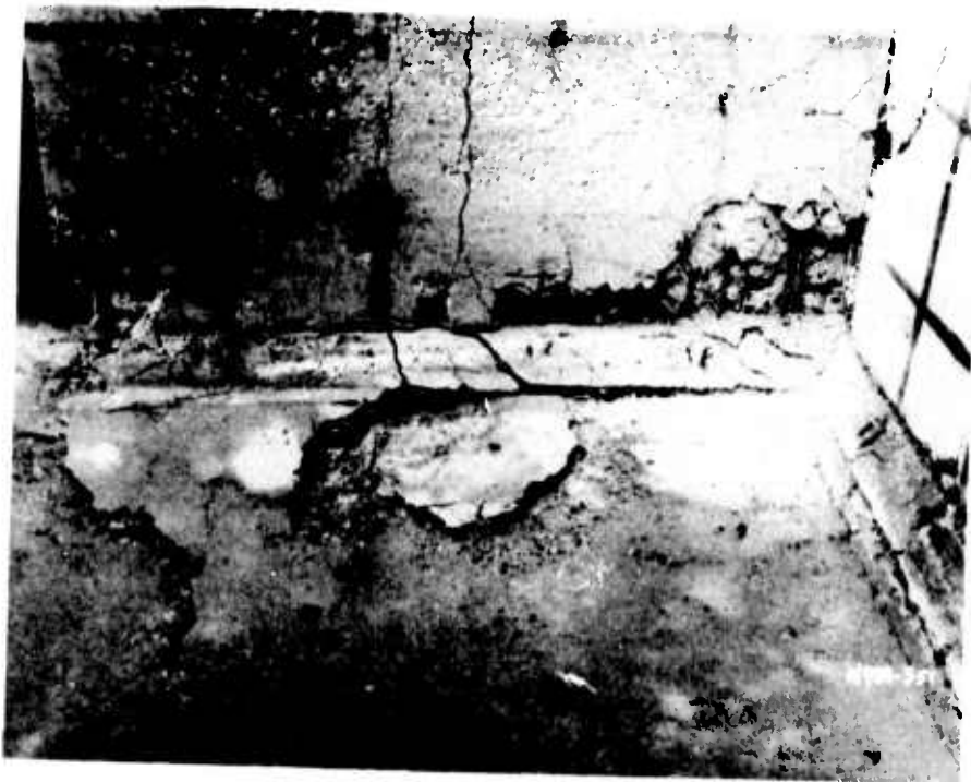
b. Damage to lower north corner.
