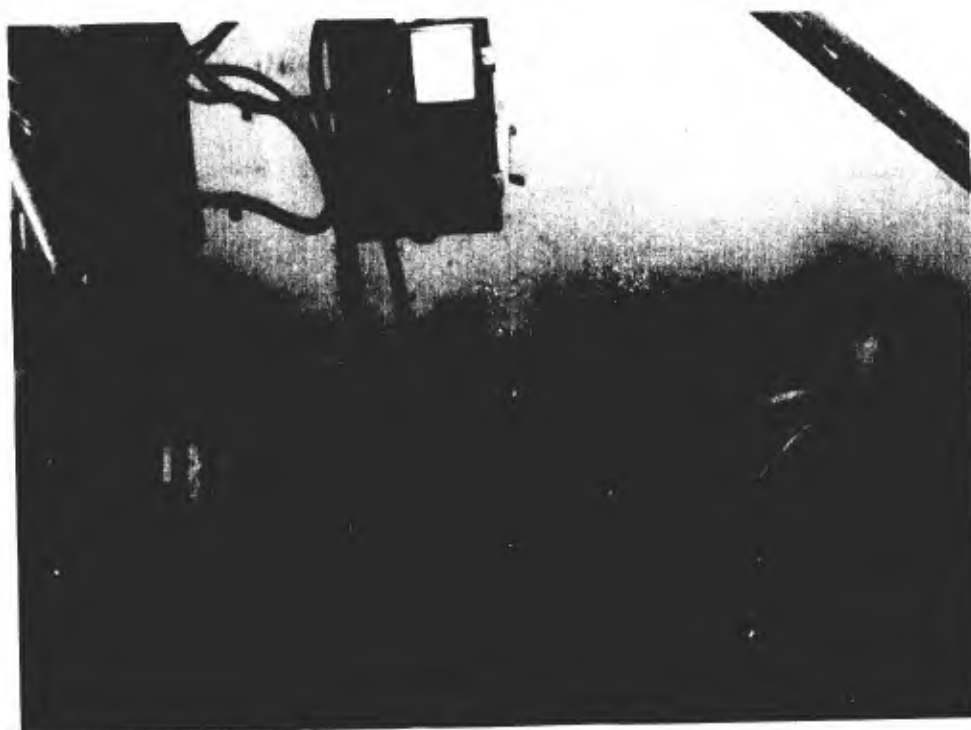
(b) Wanlass Motor Installation
