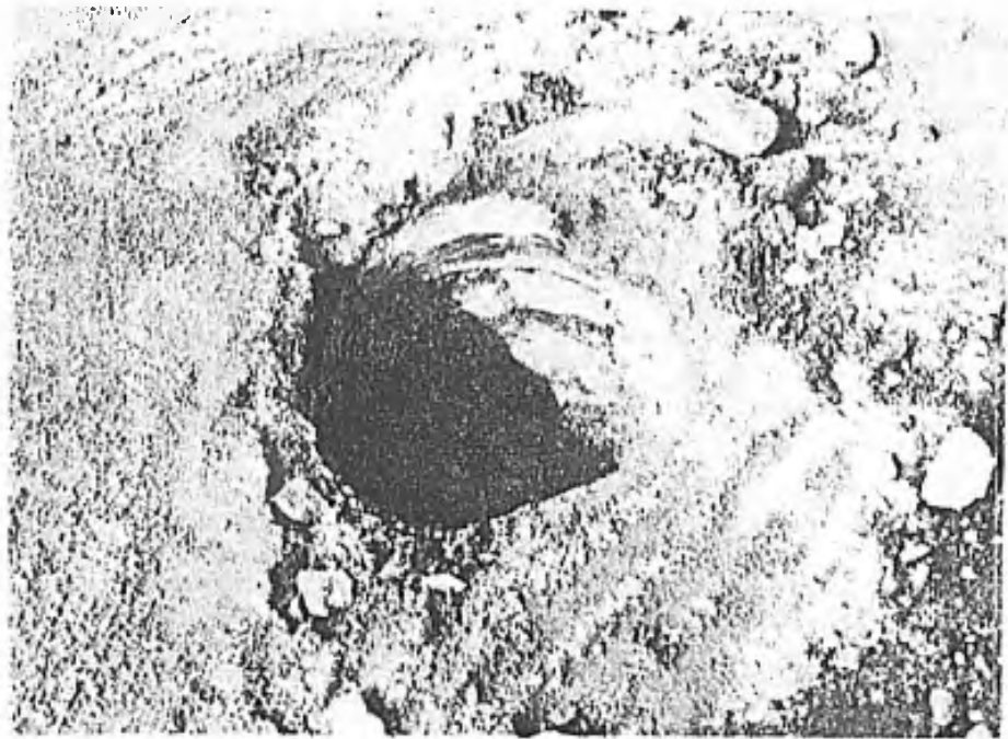
Photo 16. Top Layer (Second Lift) of the Stabilized Soil Through a Core Hole.
