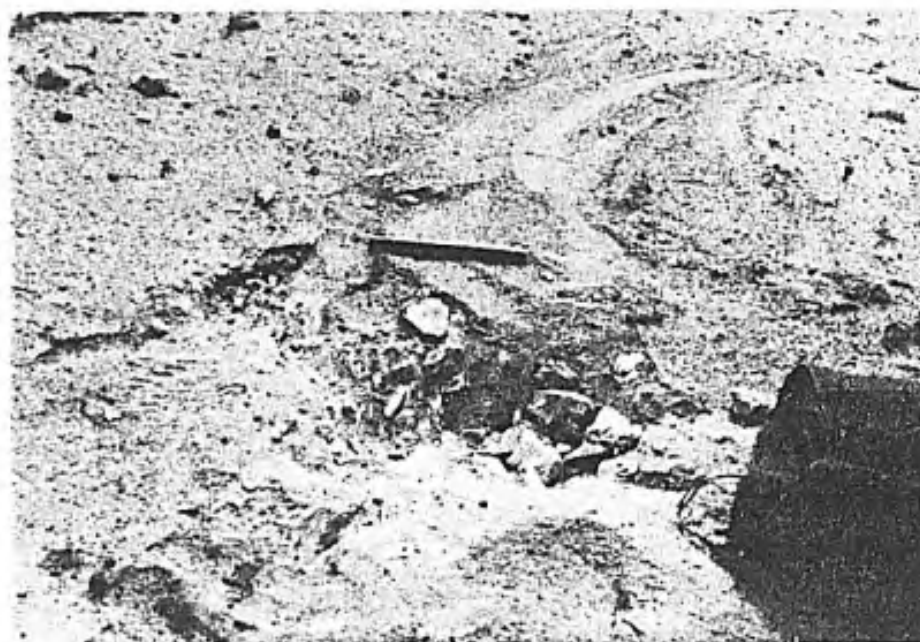
Photo 2. Damage to a Slab From a 3.5-pound Charge of TNT.
