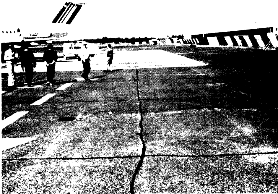
Photo 5. Reflective joints in 1976 Salviacim pavement
