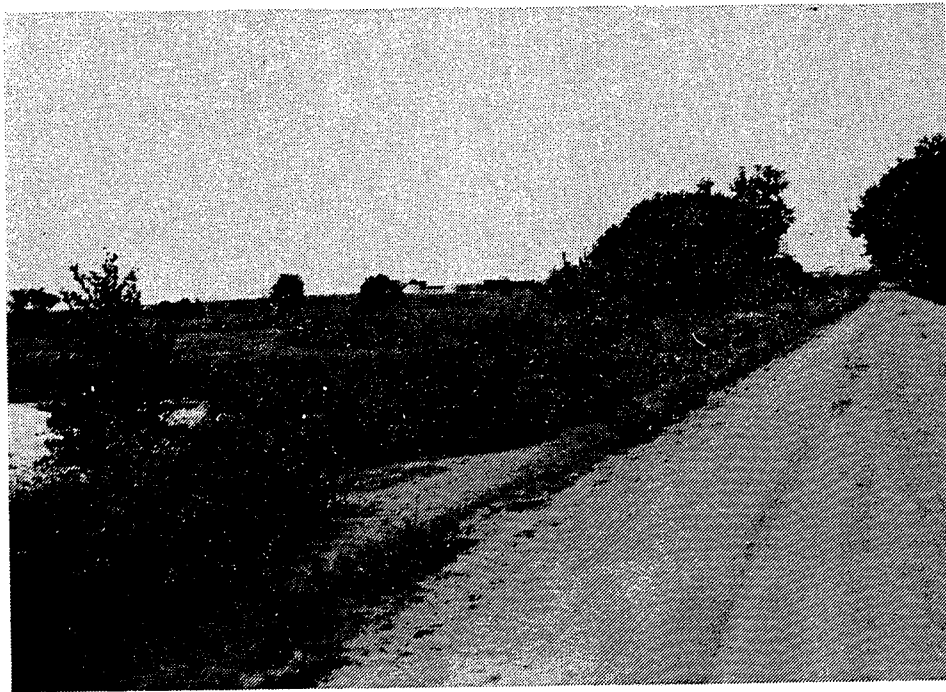
DIKE BETWEEN LOWER AND UPPER DERBY LAKE: Looking North Date of Photograph: 26 August 1982
