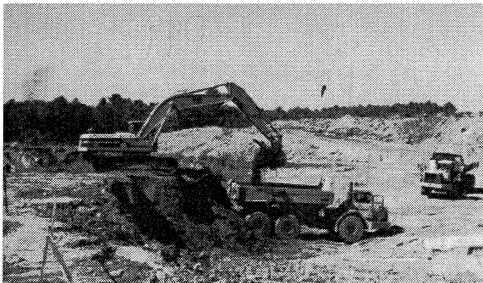
Figure 3.2: Landfill Excavation (below) and Soil Removal Project (page 30), Pease Air Force Base, New Hampshire.
