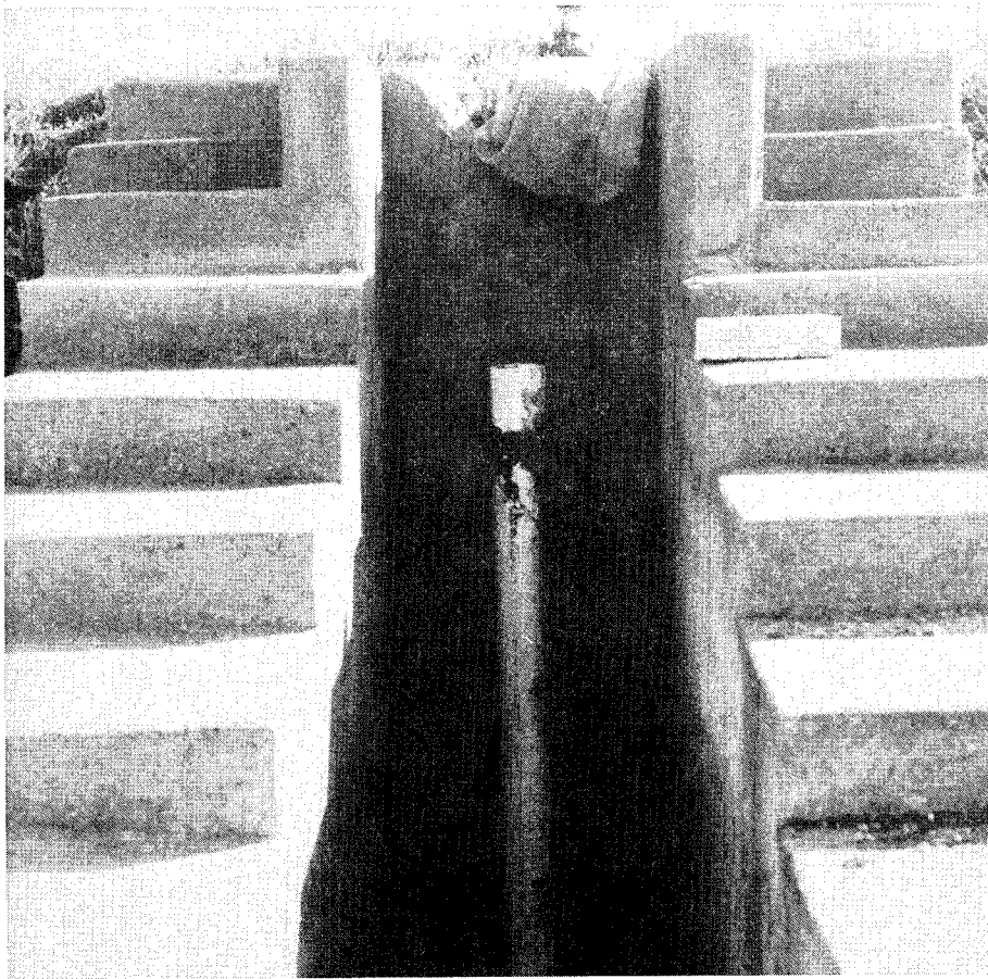
Photo 2. Stand-pipe drain in a typical LAERF pond
