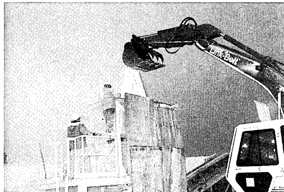
Figure 5. Direct lime feed into the weigh batch hopper.
