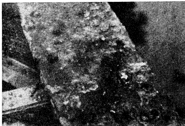
Figure 190. Corrosion of the top flange of a girder on the Santa Fe Railroad (from Hyma 1979)
