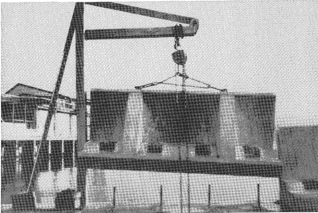
Figure 137. Precast wave deflector unit being placed by chain-block crane at Clyde Quay (from New Zealand Concrete Construction 1991)
