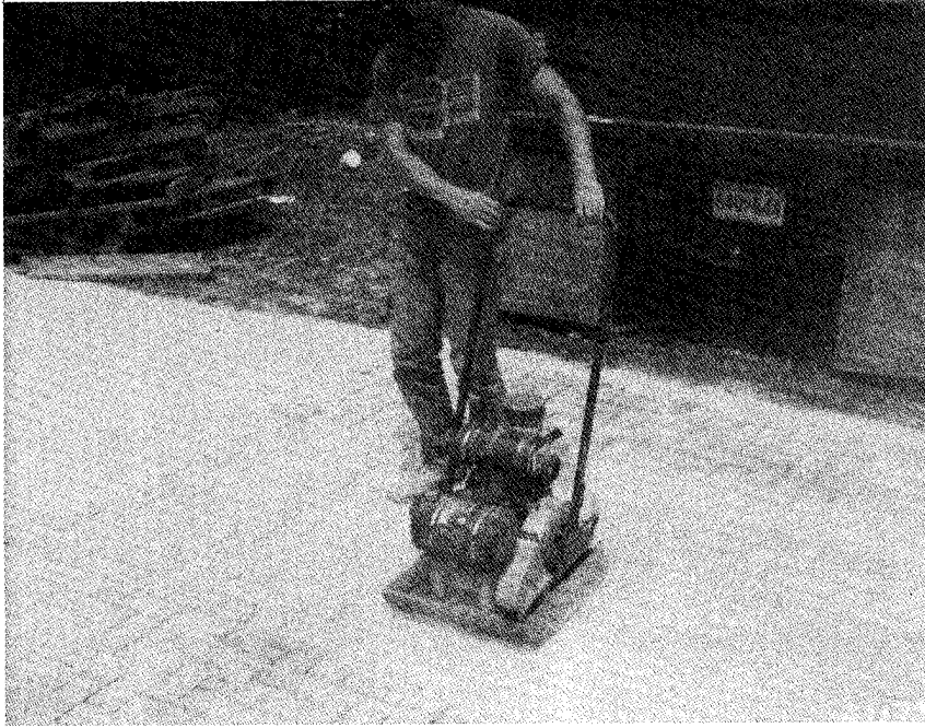
Figure 225. Plate compactor being used to vibrate jointing sand into paving block joints at Aberdeen Proving Ground (from Anderton 1991a)
