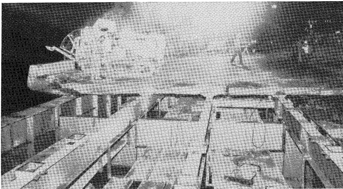
Figure 163. Painted steel and forms for bearing pads placed on stringers in section where concrete has been removed, Woodrow Wilson Memorial Bridge (from ASCE 1984)
