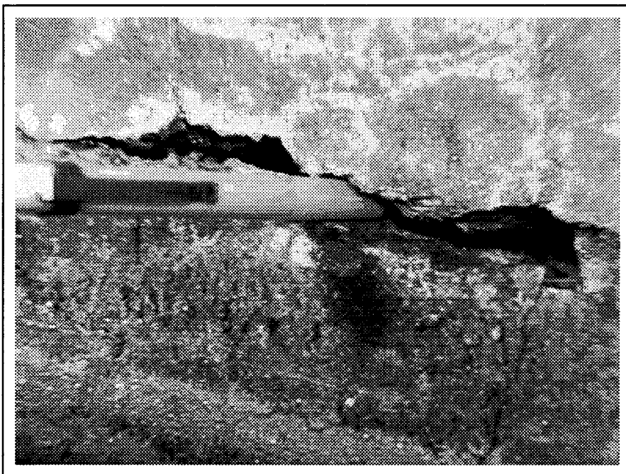
Figure E2. Closeup of burner refractory damage.
