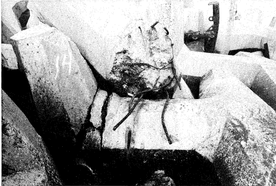
Figure 21. Dolosse on north jetty with shank-fluke breaks
