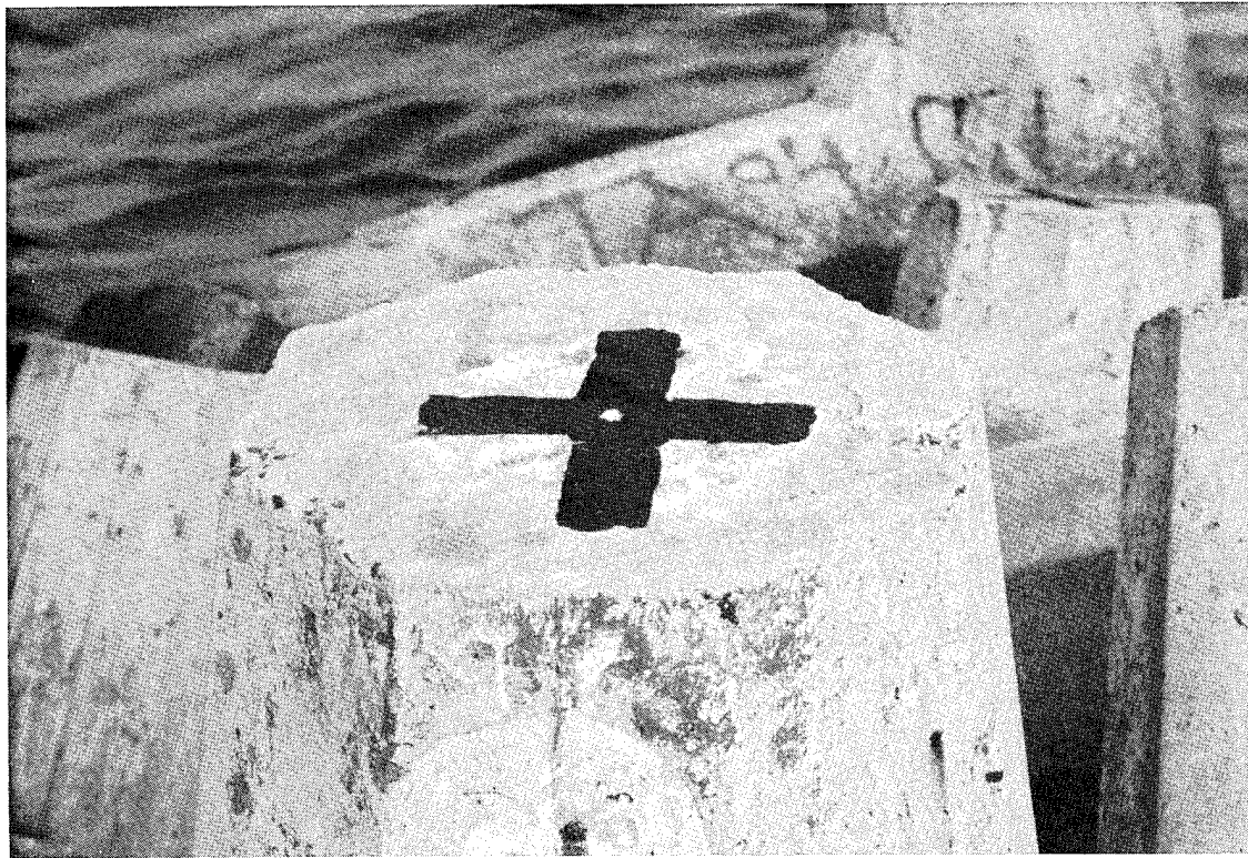
Figure 15. Typical target established on a dolos armor unit
