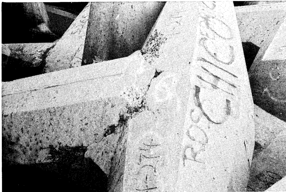
Figure 20. Dolos on south jetty with shank-fluke crack
