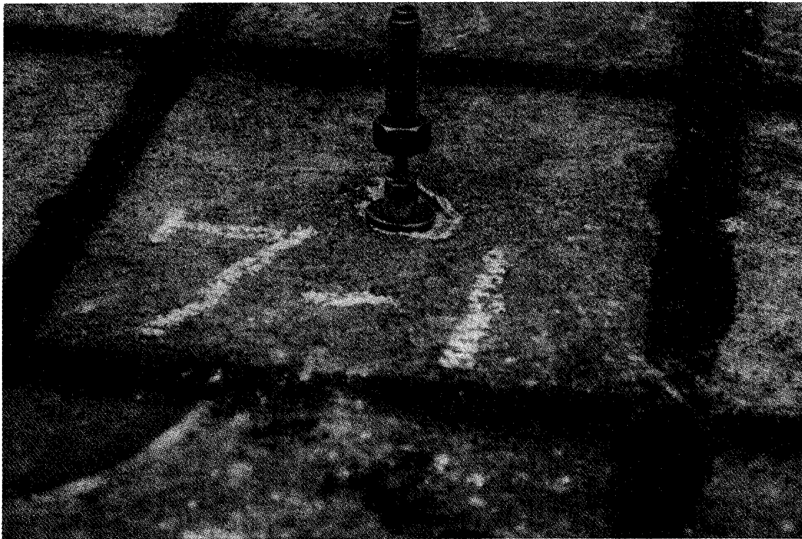
Figure 30. Pullout failure of impact set anchor. The anchor displaced approximately 1/4 in. and then the steel failed in tension
