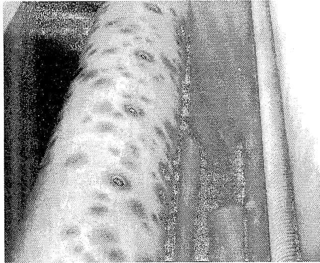
Figure 4: HV damage to G-11 tube.
