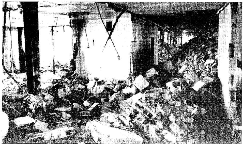
Figure 2. Clay tile partition rubble from 1979 renovations
