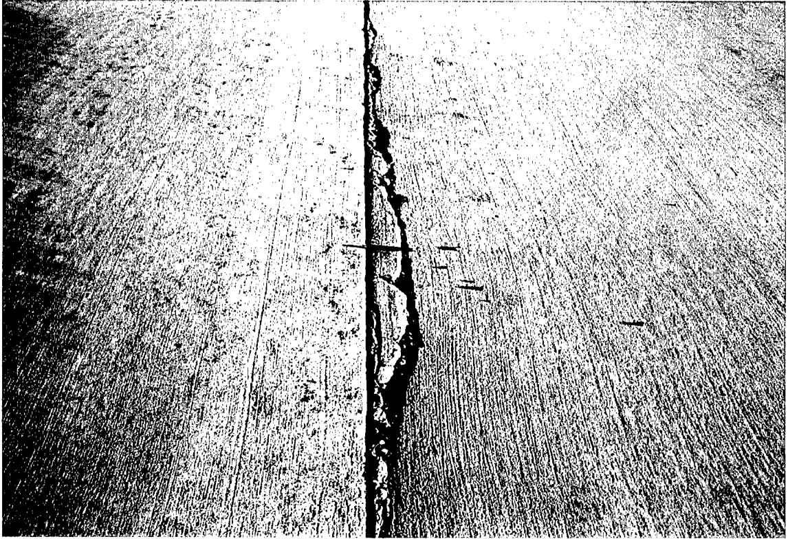
Photo C9. High-severity joint spall on the Parking Apron
