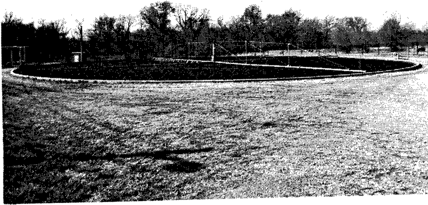
Figure 109. Building 2203: Sewage Sprinkler Filters.
