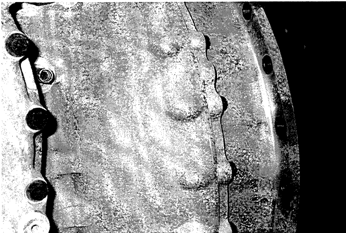
Corrosion Occured Due to the Water Based Solvent
