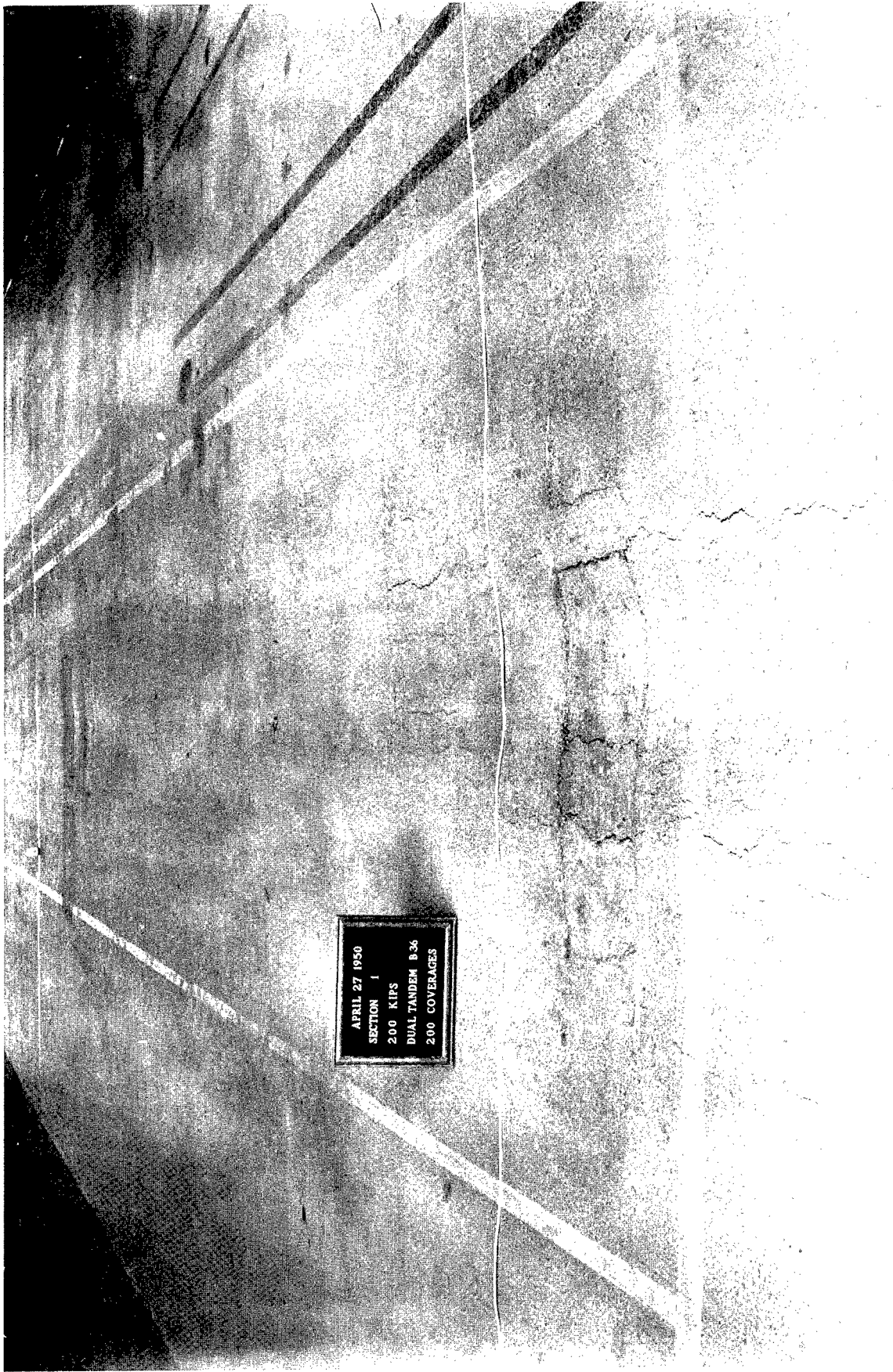
Photograph 10. Unit 1, 14-in. thickness. View showing rutting and failure after 200 coverages with 200,000-lb load on B-36 assembly
