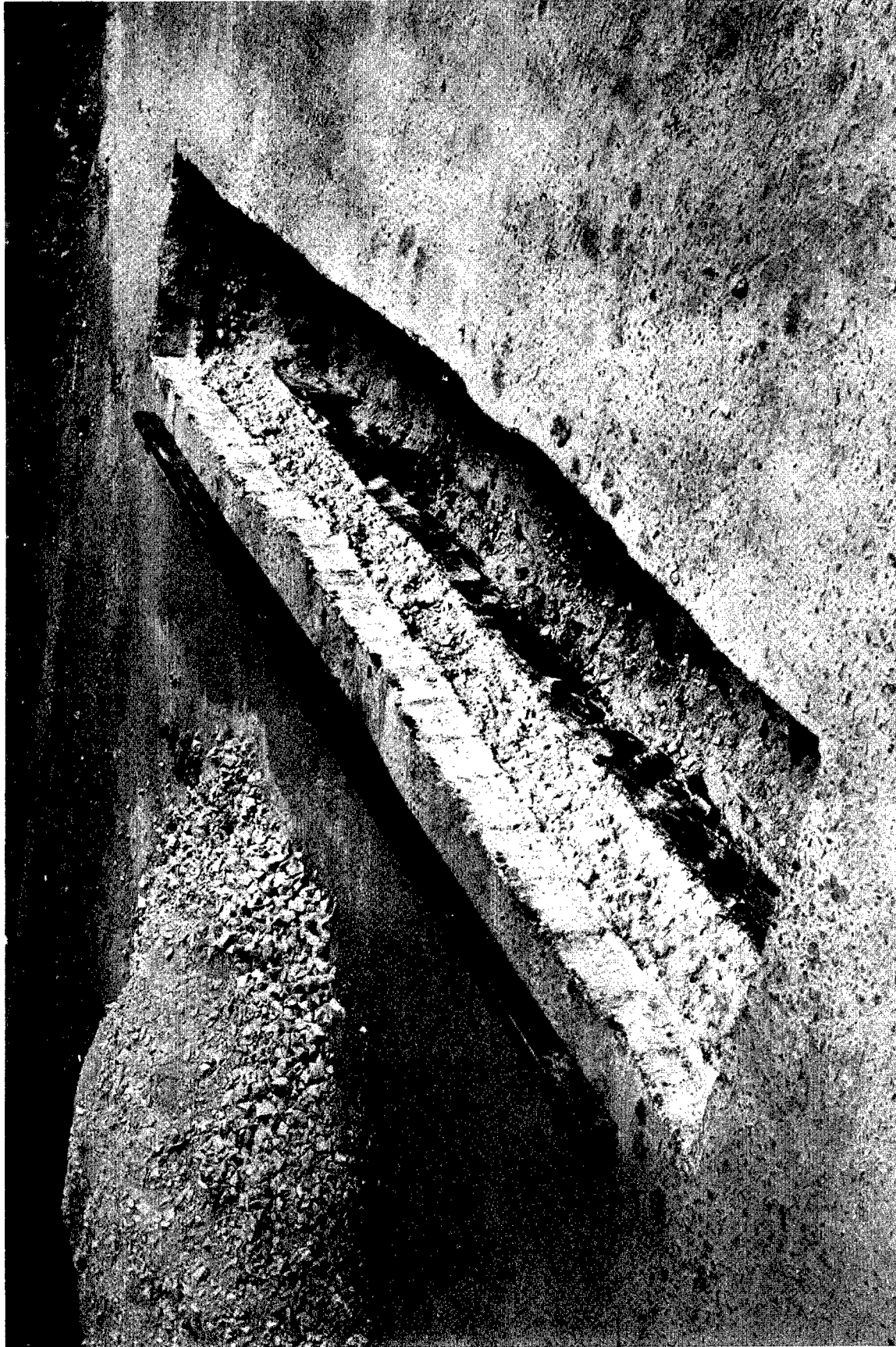
Photograph 15. Unit 4, 10-in. thickness. View of pit 4 after 2,000 coverages with 70,000-lb load on B-29 assembly
