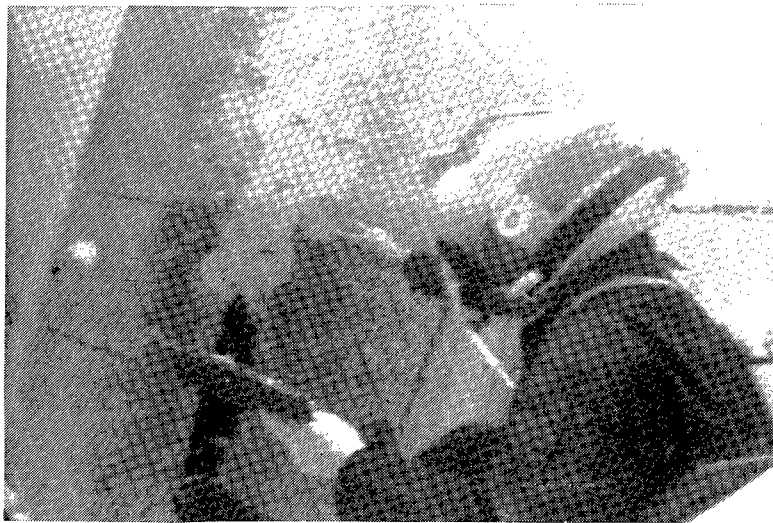
Figure 27. Surface preparation compound being applied to rough concrete at perimeter of repair area
