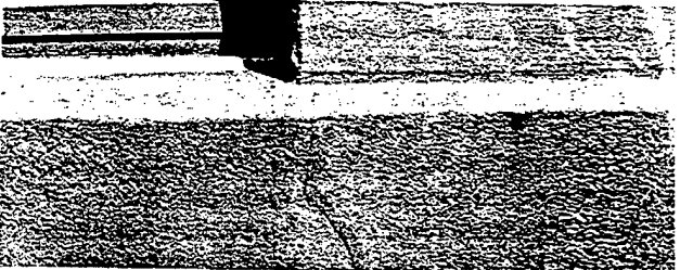
Fig. 13h. This active crack at a window sill and in the foundation wall has been filled with a flexible sealant. This area was subsequently painted with a masonry paint compatible with the sealant.
