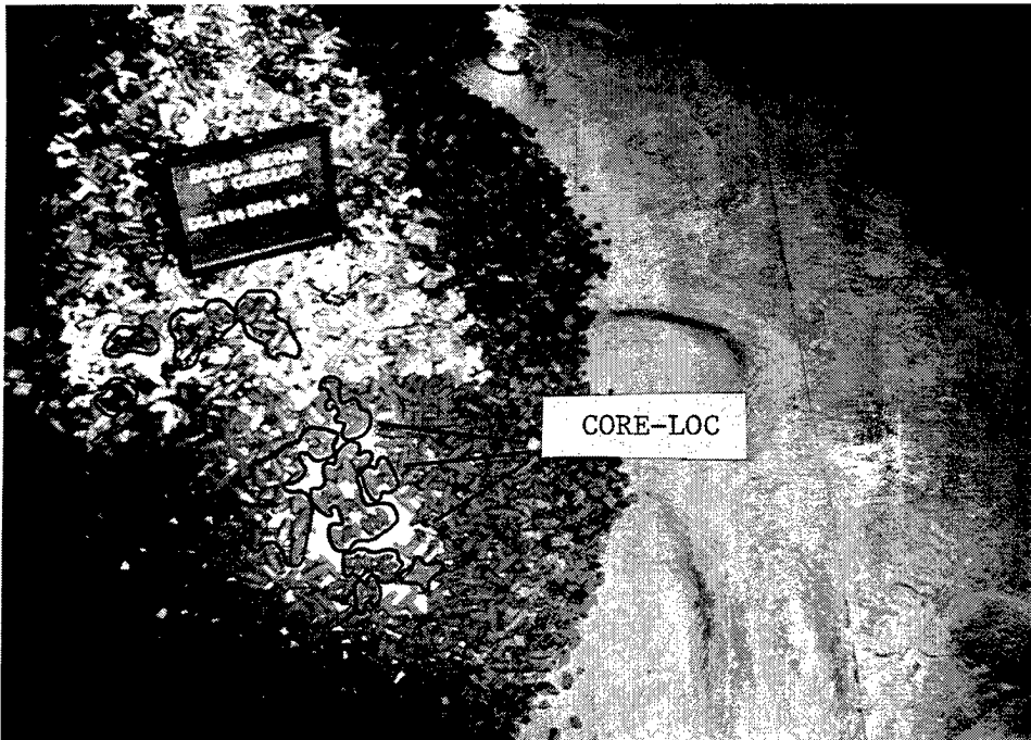
Photo A8. TS3, damage to Core-Loc repair after 2 hr
