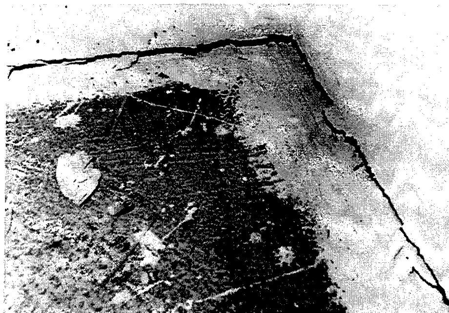
Figure 32. ITS-1, close-up view of interior south-east corner, imposed top deflection of 2 in.
