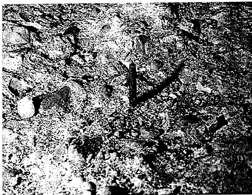
Figure 80. ITS-2, typical failed reinforcing bar.
