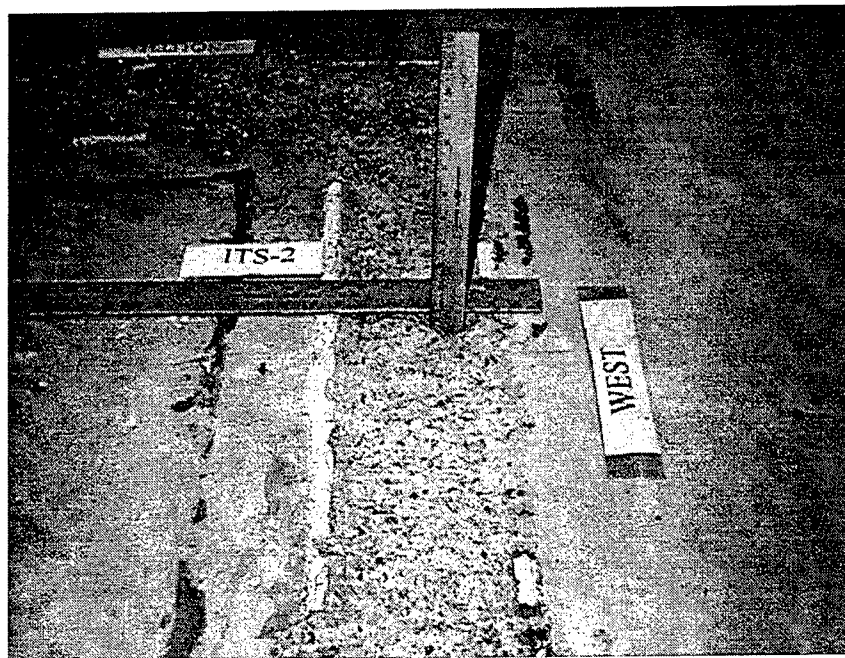
Figure 79. Close-up view of failure plane under west wall of ITS-2.
