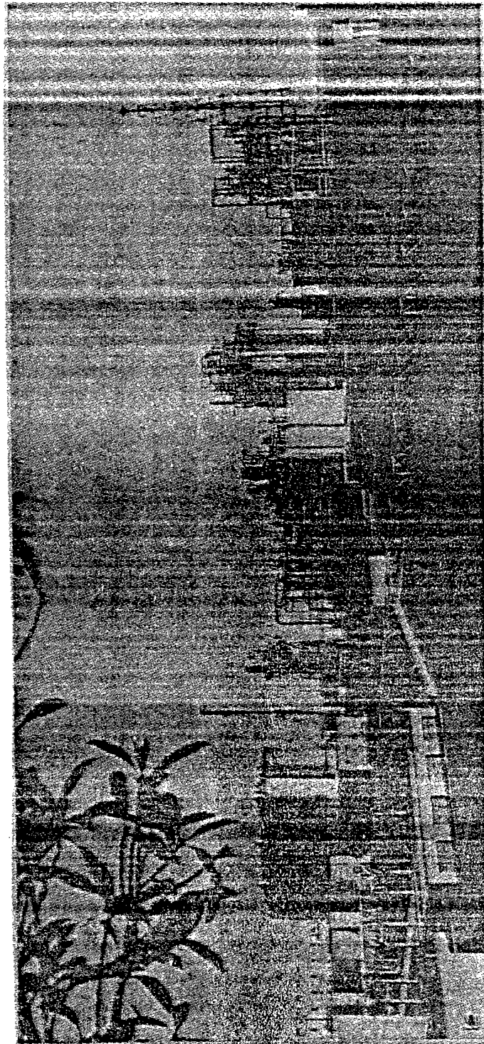
Fig. 2 A view of the polyester facility being built at the Shanghai General Petrochemical Plant. Upon completion, the imported installation will turn out 200,000 tons of dacron raw materials annually.
