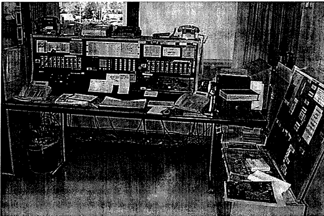
Figure 22. Equipment at emergency room communications center resting loosely on a table.
