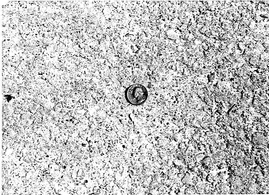
Figure 37. Surface deterioration of Material No. 12C (Illinois)
