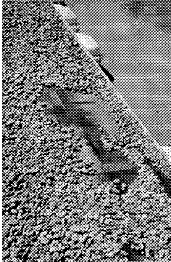
Figure 6. Failed patch along the north edge of roof D1, looking NW.
