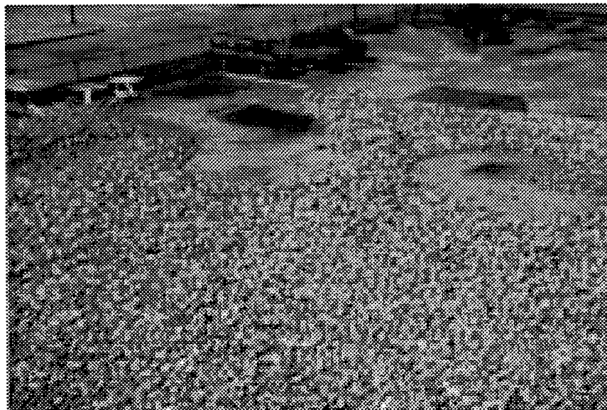
Figure 4. Ballast scour in the northeast corner of roof D1.
