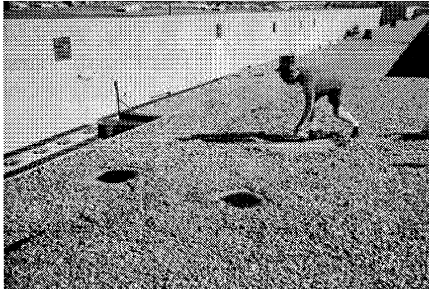
Figure 8. Southeast corner of roof D1 showing areas cleaned for cores 1 and 2 and a larger area being prepared for core 8 and cut A, looking SE.
