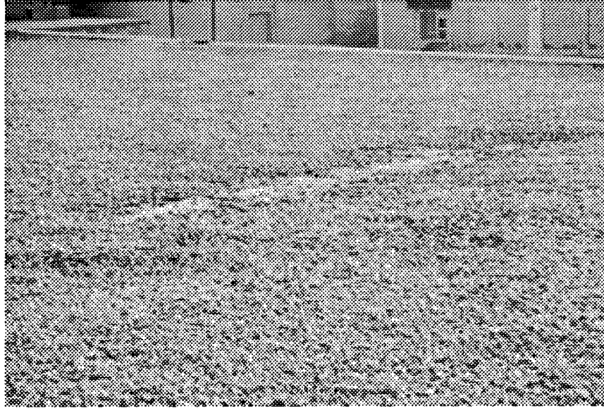
Figure 19. Bare area on roof D5, looking southwest.
