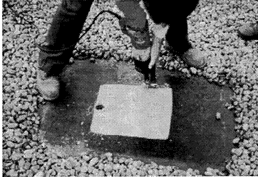
Figure 22. Hole where core 5 was taken and where cut E is being taken on roof D6.
