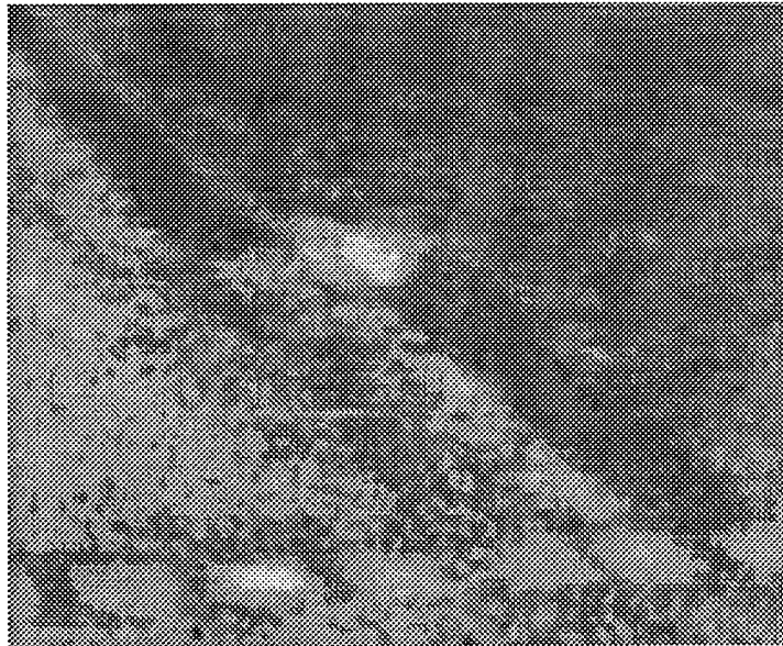
Figure 28. Photograph and thermogram of the expansion joint that separates roofs A2 and A3, looking a little south of east. The bright spot on the thermogram suggests that wet insulation exists below the patch.
