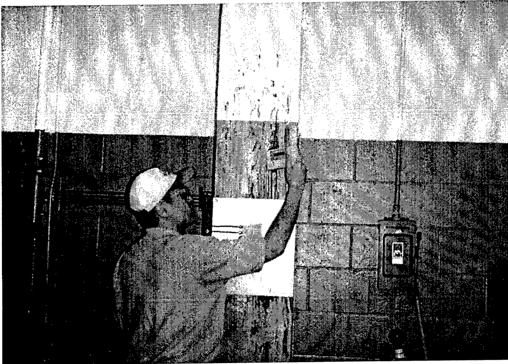
Photo 23. Using the moisture content meter on termite damaged column.
