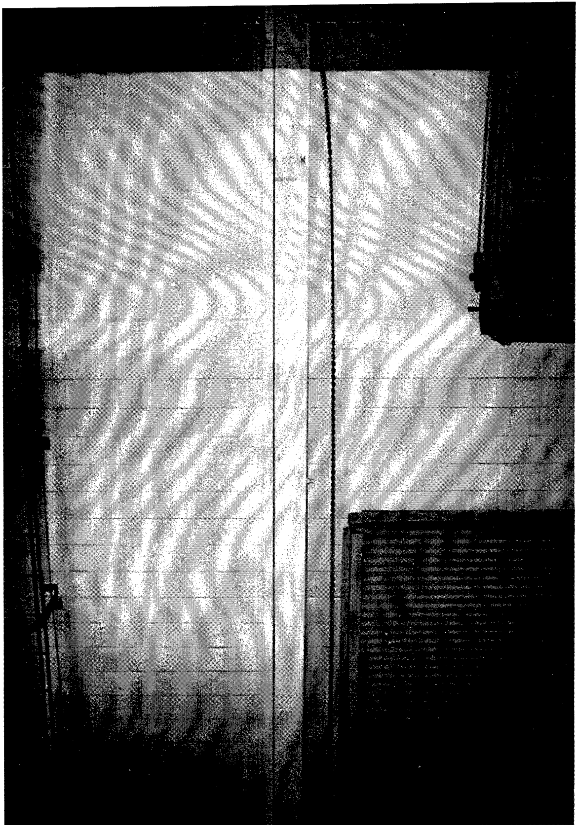
Photo 2. Misaligned slender column with loose bolts.
