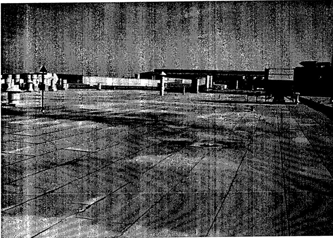
Photo 19. Water collected on the roof surface of Area B.
