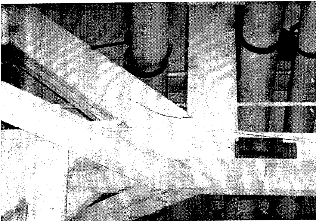
Photo 28. Fracture on member CT of column line 63.
