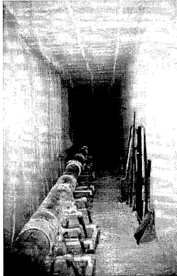
Figure 20. Extended ducts in tunnel.
