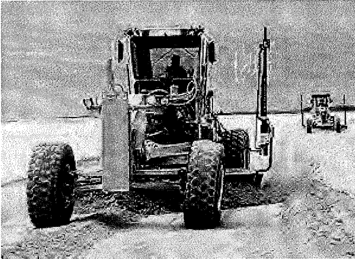
Figure 12. Manual Grader Laser Control System (TOPCON Laser Systems, 1999)
