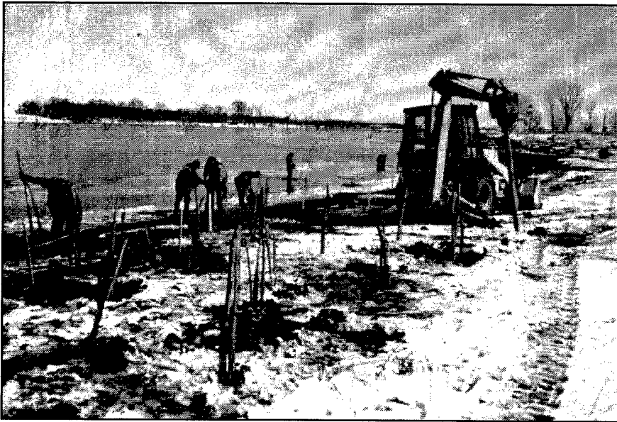
Figure 4. Dormant willow posts being installed with the aid of a backhoe mounted with a "stinger"
