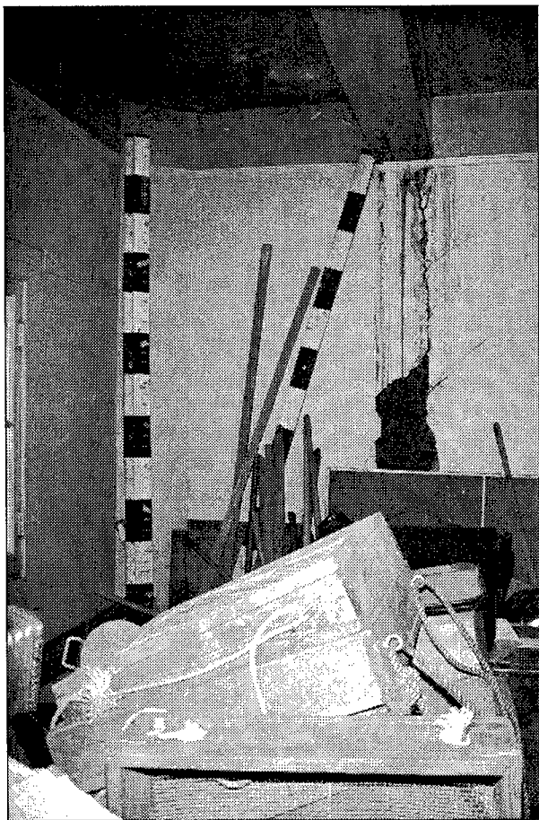
Figure 39. One wall of the collections storage area in Storage Location 2 has been damaged by water. Note also the piles of miscellaneous equipment cluttering the floor.
