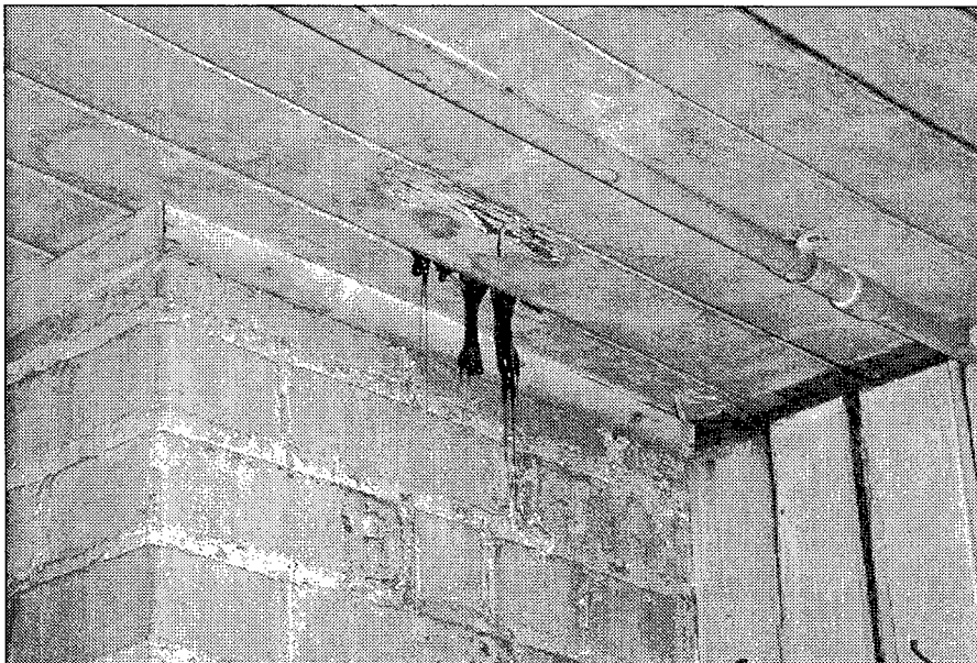
Figure 22. Dried tar (leaked from the tar and asphalt roof above) hanging down from the ceiling in the collections storage area at GCM Services.
