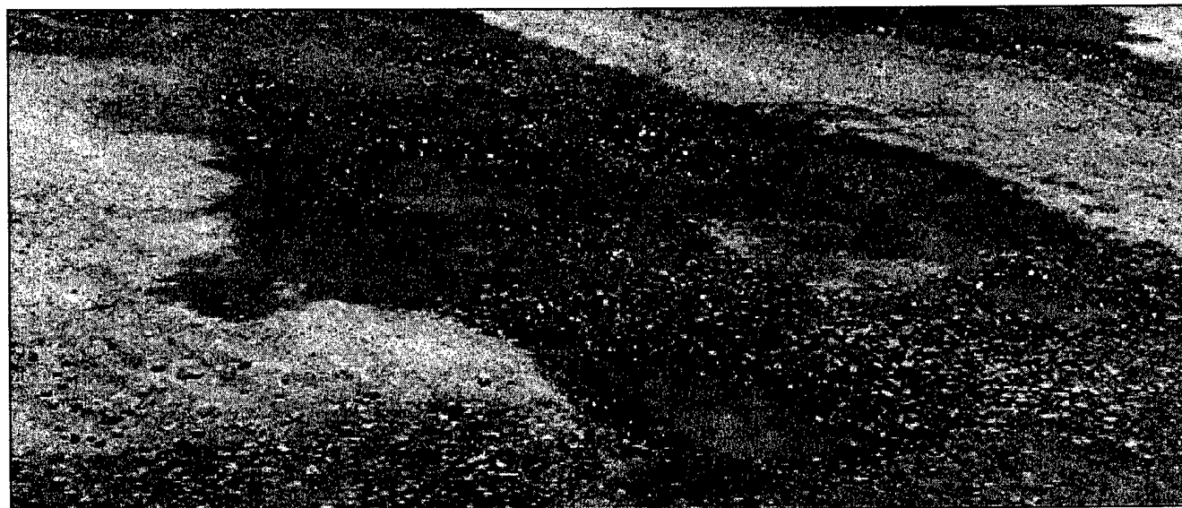
Potholes in Road Base
