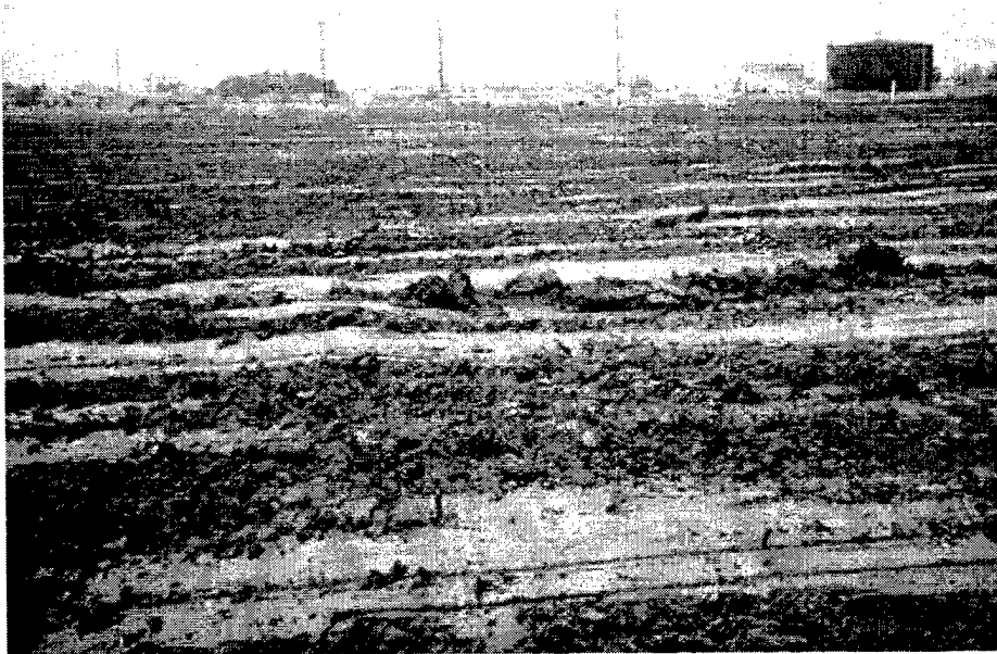
Figure A1. Freshly placed, Portland cement processed material at the Jersey Gardens Mall Site, Elizabeth, NJ
