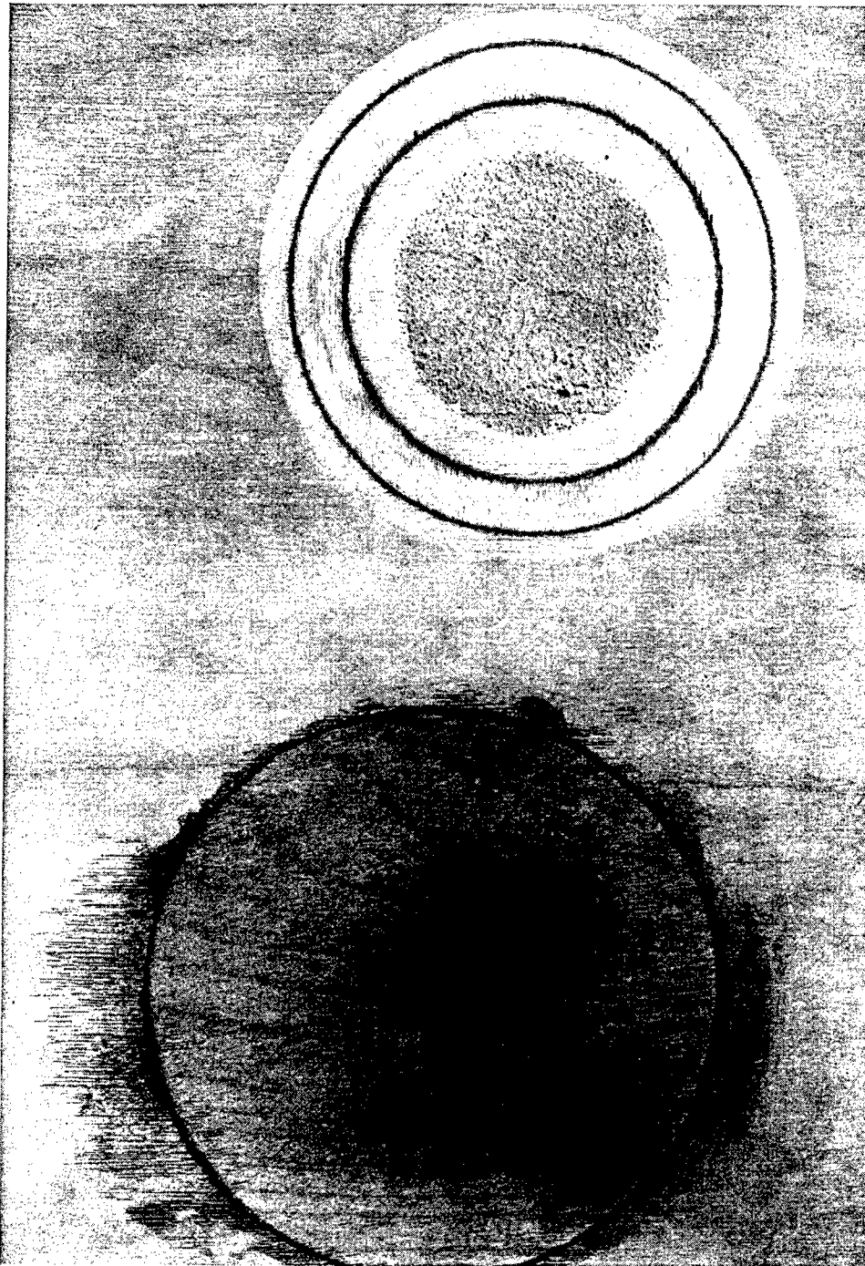
Figure 7-14. A small inlay recess (top) and completed inlay repair (bottom) in plywood-faced sandwich.
