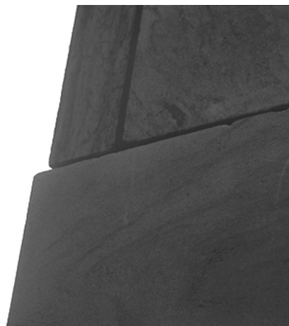
Figure 6: Stone Displacement Due to Effects of Age
