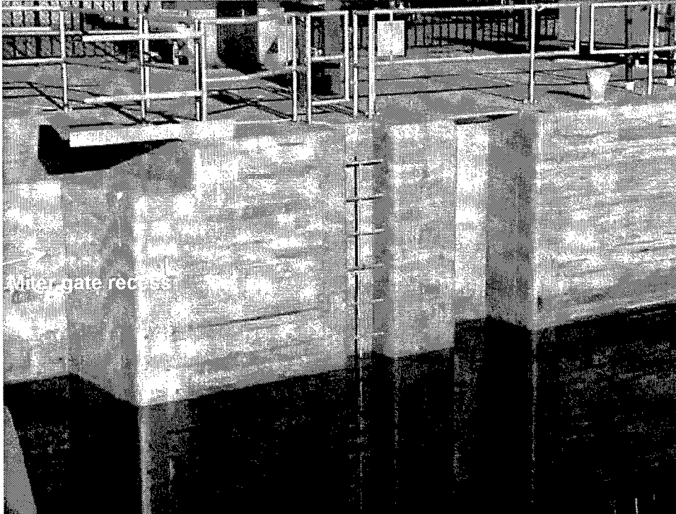
Figure 3. Upper pool water level pressure transducer location
