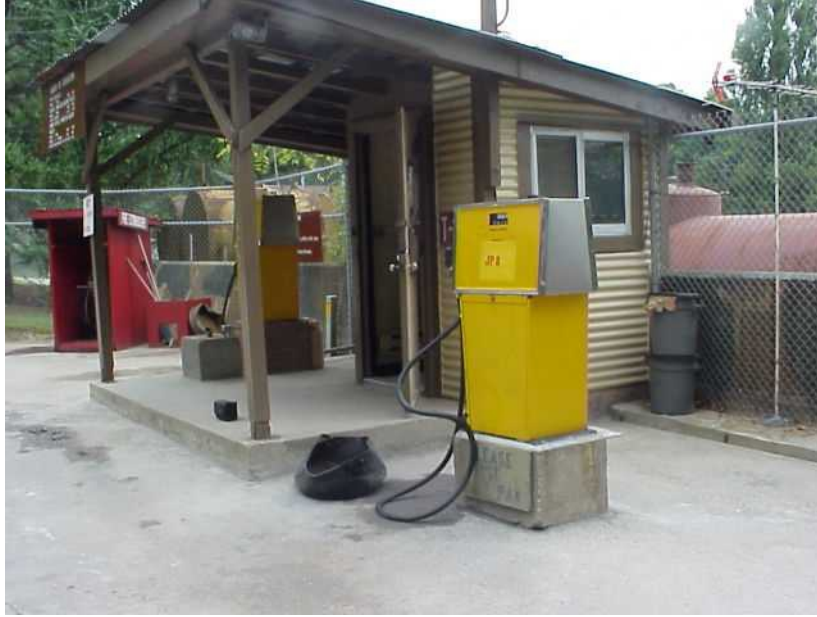
Figure 26. JP-8 Dispensing Pump
