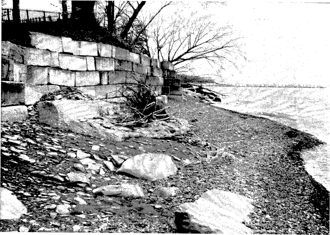
Figure 17. Concrete block wall about 200 m east of marina, 17 May 1991. Leaning tree is seen in subsequent figures
