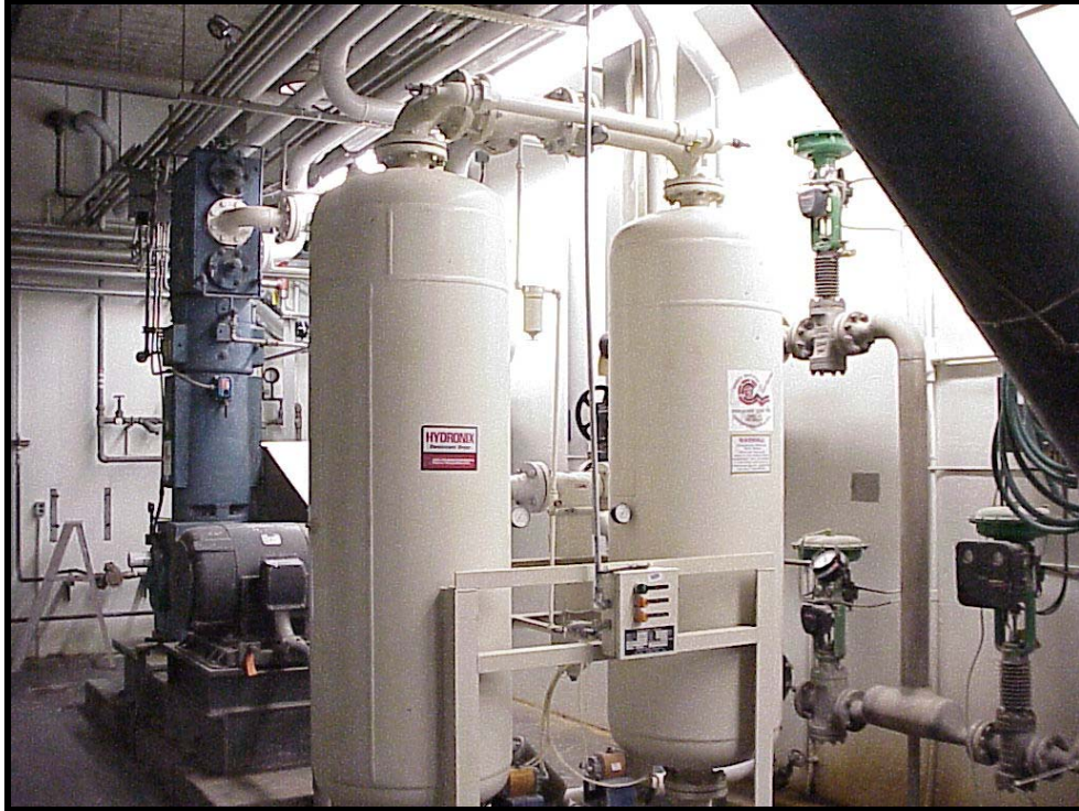
Figure 2.3. Hydronix desiccant dryers (in parallel).
