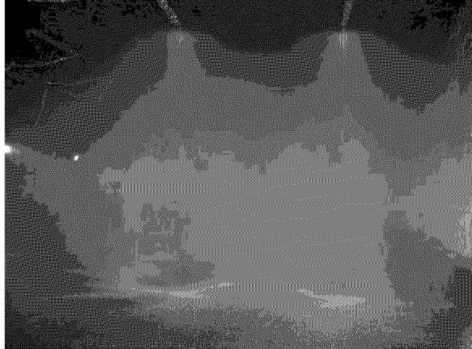
Figure 5: Four Discharging Sprinklers
