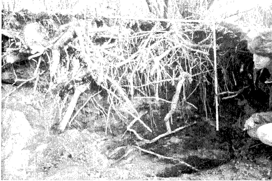
Figure 4. Shallow rooting depths of grasses are less effective at stabilizing banks than deeper rooted trees and shrubs
