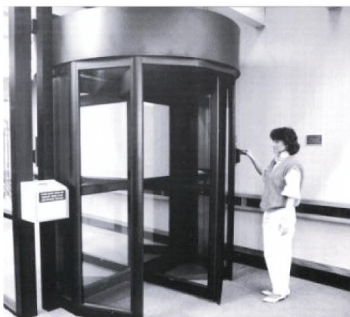
Revolving doors begin to turn as soon as card reader successfully scans an employee's badge.
