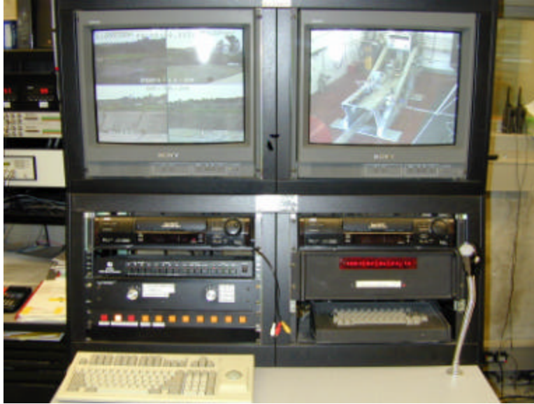
Figure 10. Control Room Operations Panel
