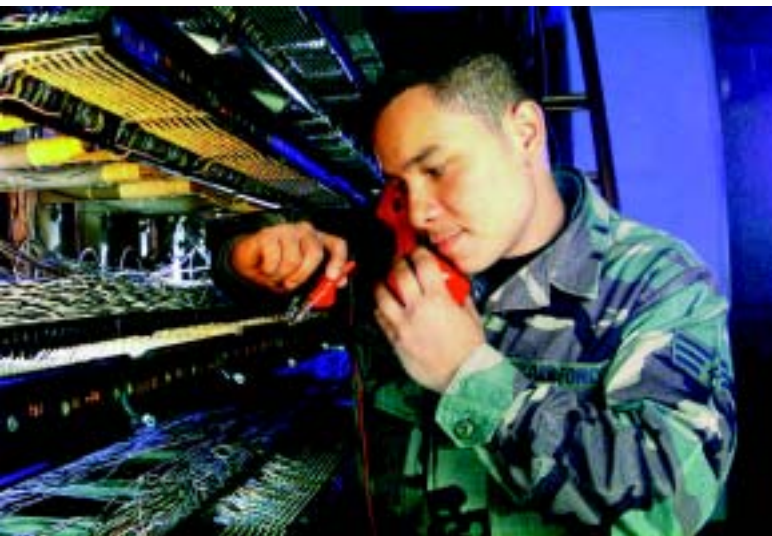
Our personnel are working hand-in-hand with commercial utilities to privatize 434 Air Force utility systems.
