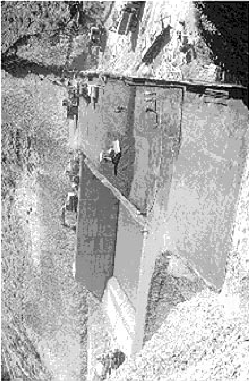
Photo C-4. Placing RCC lifts at elevation above the top of the training wall
