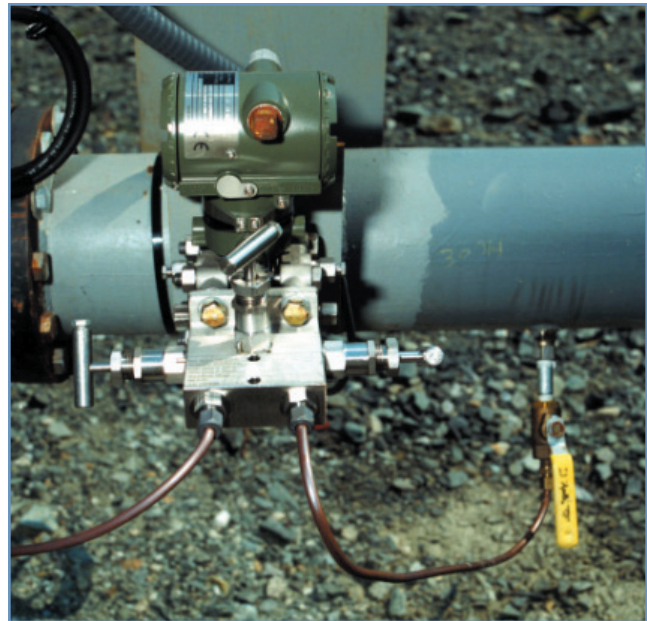
Figure 2. Differential pressure sensor installed next to an isolation valve.
