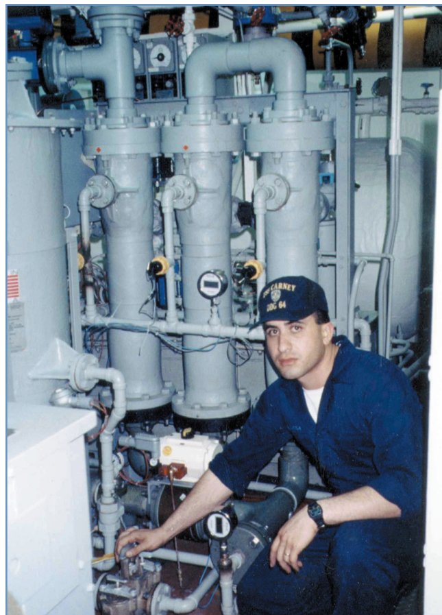
Figure 3. Prototype 10 gpm oily waste membrane system installed aboard USS CARNEY (DDG 64).
