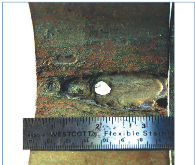
Figure 1. Localized corrosion in forward drain system piping.
