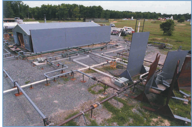
Figure 5. Aerial view of the fire main piping system and the test site.
