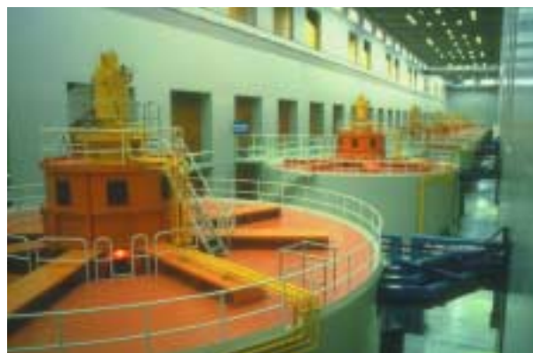
Turbines inside the Bonneville Dam powerhouse, Oregon.
