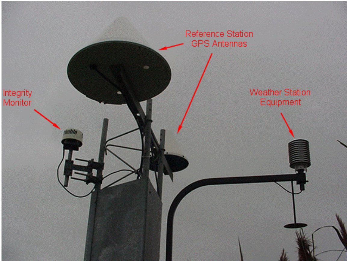
Figure 68 Typical USCG DGPS Receiver Antenna Layout
